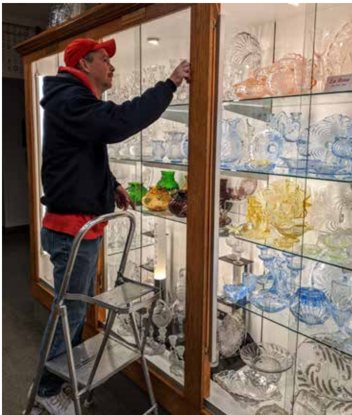
The new vertical LED case lights look wonderful. Ben Kirkman has done a great job with the installation and ballast removal.
