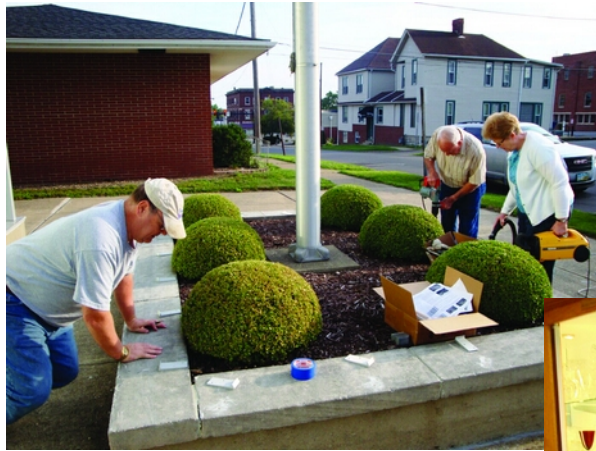
Museum volunteers (L-R) Larry Everett, Carl Beynon and Susan Everett work on installing skateboard deterrents on the planter in front of the museum. The planter had been waxed by skateboarders that were using it in the evening and the surface was deteriorating. Since the deterrents were installed they haven't used the area again.
